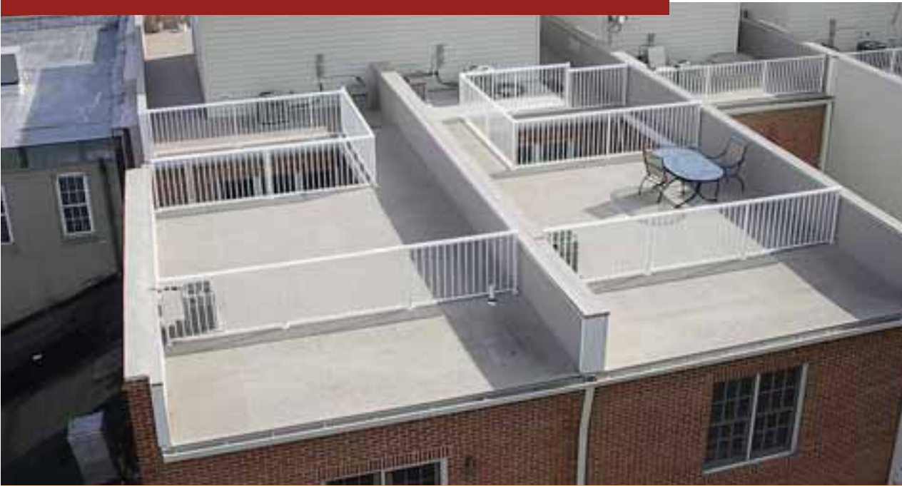
PVC membranes were specified for roof decks at a Baltimore-area town house development. Bond Street Townes, Fells Point, Maryland. Architect: Architecture Collaborative, Inc.
