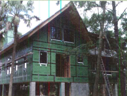
Acrylic tape helps prevent drafts and potential moisture intrusion in the above project, similar to HGTV's Dream Home 2013.
