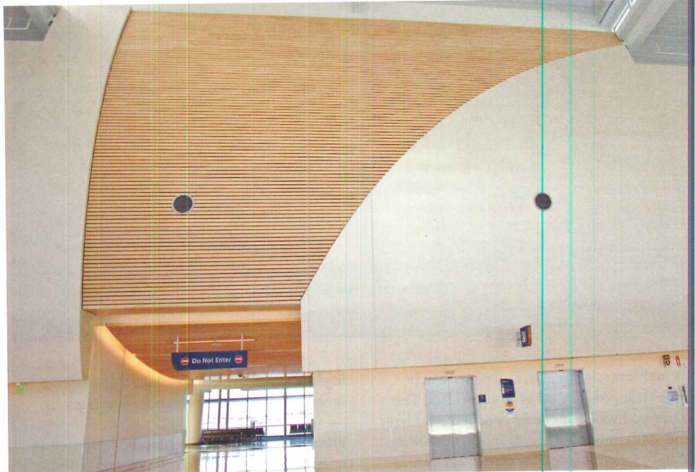
Photo courtesy of Hunter Douglas Contract
