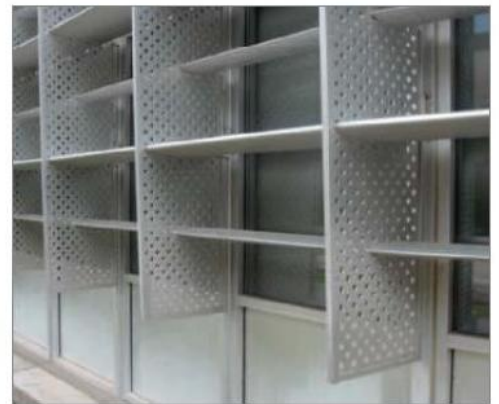
EASTERN ARIZONA COLLEGE 8" & 17" airfoils inside perforated vertical fins
