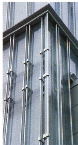
Steel wind clips and staggered shelves hold the glass channels in place (above), and a layer of shiny aluminum siding sits behind the glass.
