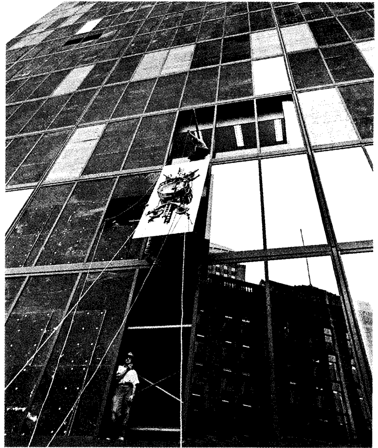
Reflective glass panels on Boston’s Hancock Tower fell during a windstorm.
