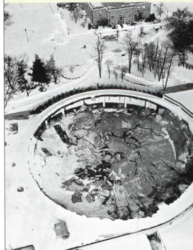
An aerial view shows a frighteningly thorough collapse of the C.W. Post Dome.
