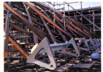
The MoMA arch began with four- to five-inch diameter tubes (top). These were preassembled and lowered into place by crane. The arch rests on the ground and is tied to the museum wall (bottom).
