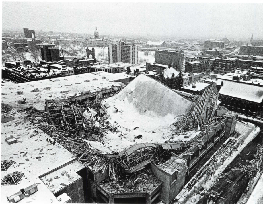
The roof of the Hartford Arena collapsed in January 1978 under the weight of a heavy snowfall.
