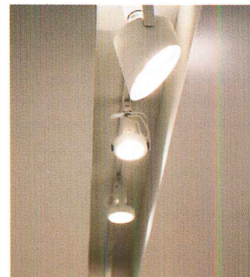
Monopoints can be plugged in along the beams wherever they are needed (top). A channel in a ductwork soffit hides track lights (above).
