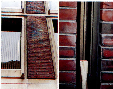
An example of a location requiring a fillet joint (left) and application of new sealant over old (right).
