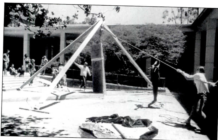
UCLA students reconstructed a section of the King's Road House using Schindler's innovative lift-slab technique (bottom photo). Schindler and his partner are shown building the original (top).
