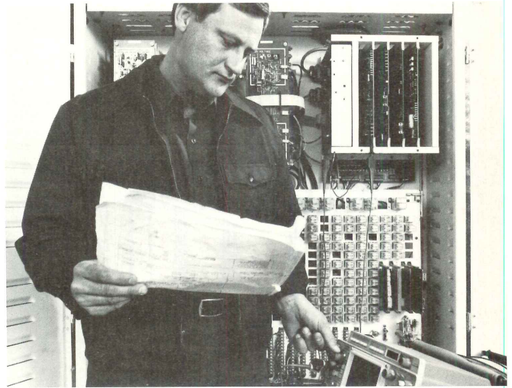
controls. Increasingly, elevator maintenance is enhanced by computerized control monitors that store data about each elevator's performance and possible malfunction.
