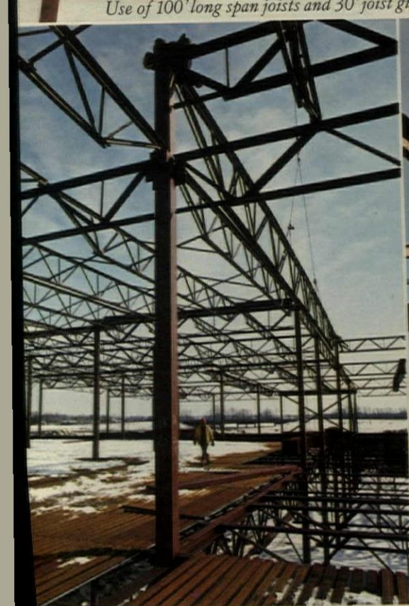
Wide spacing of deep steel joists (6'8" in floors and 7'6" in roofs) resulted in stiffer floor system and saving in the cost of joists.
