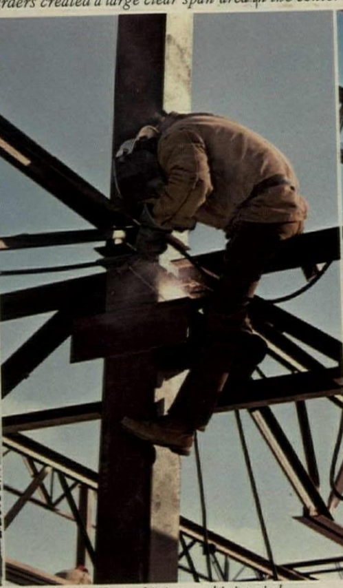
Vulcraft steel joists and joist girders allowed for simple and fast column connections.
