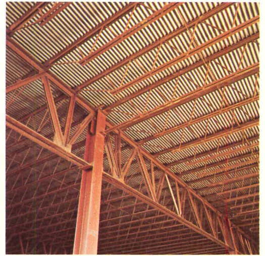
Joist girders have top chord panel points that show joist location. Which makes a lot of measuring unnecessary.
