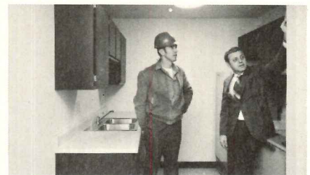
Hide-A-Spray paint dried in two hours. Contractor installed cabinets and floor covering the same day. Walter Scharfe, left, Job Superintendent for Lloyd Construction, commented, “Conventional two-coat paints would have meant a week’s time between painting and any such installation.” PPG Paint Center Manager, Eugene Lee, is shown at right.
