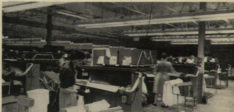
GE Power Groove fluorescents boosted the light in this textile factory. And production shot up 15%.
