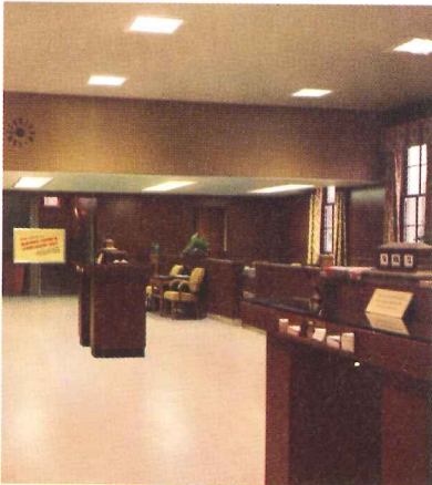
Spectra V luminaires for this savings and loan office. The 400 watt luminaires were easily installed in the T-bar suspended ceiling. For visual comfort Low Brightness models were chosen. Recessed or surface-mounted units available.
