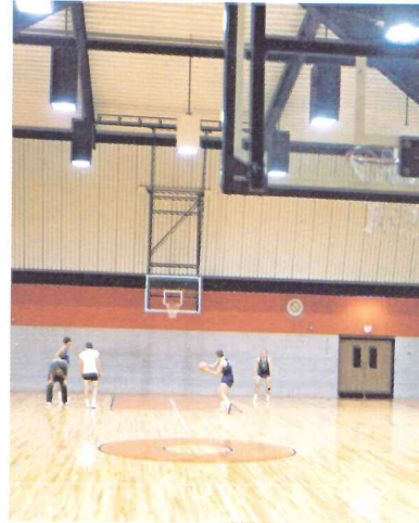
Twenty Spectra VI pendants provide an average 81 footcandles of uniform lighting in this gym. These rugged but handsome fixtures are available in 400 and 1000 watt models.
