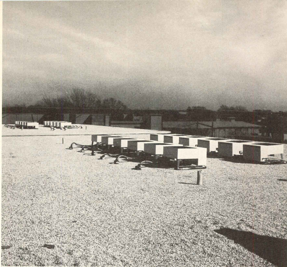
Mi Amigo Apartments, under construction in Dallas, is a complex of 149 apartments with individual ducted Lennox heating and air conditioning. New-design cooling units hide low on the rooftops. Architect: John Moss. Building Contractor: GTC Company. Heating/cooling contractor: Citywide Plumbing & Air Conditioning. Owners: George T. Connell and M. I. Harris, Jr.
