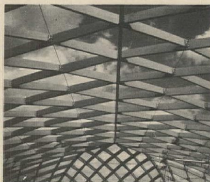
The high fire-retardance of this Pyresote® treated Lamella roof in the Mt. Vernon High School gymnasium, Mt. Vernon, Indiana, afforded substantial savings on fire insurance. Architects: Lester W. Routt & Associates; Vincennes, Indiana.
