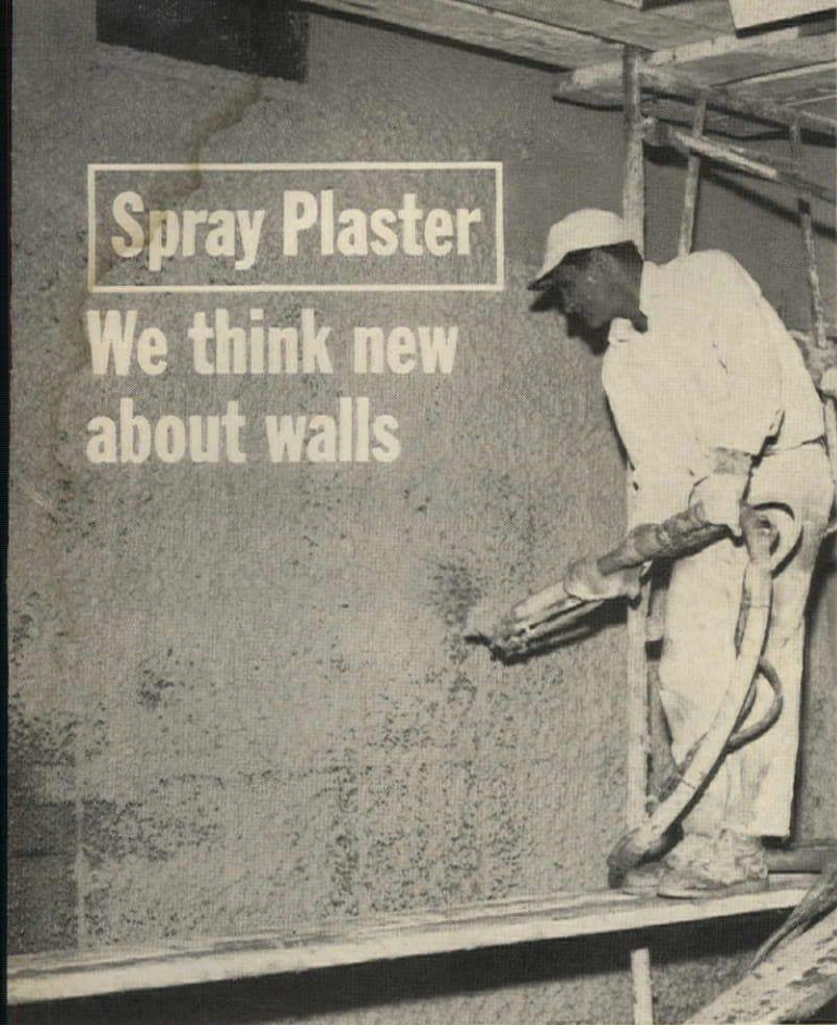
Application of scratch coat with spray machine over metal lath and steel studs.
