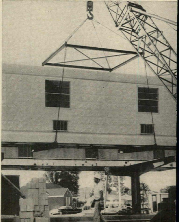
A four bedroom section being swung into position by crane. Two duplicate sections, facing a corridor, provide a total of sixteen rooms.
