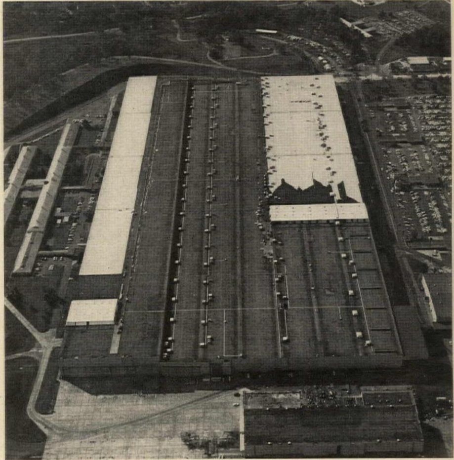
White areas are the cap sheet of the new roofing system for Lockheed-Georgia plant. Aluminum shelters protected the work and the factory interior during replacement
