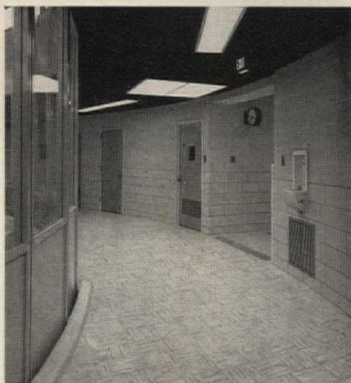
Harrelson Hall corridor shows attractive Amtico Vinyl Asbestos Floor Tile that typifies 85,000 square feet installed in curved floor plan. Principal color: Amtico AVA-204, featuring bamboo marbleization on white background.
