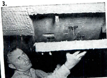
3. FIBERGLAS insulation, Type PF-613, 2" thick — bonded to concrete ceiling using MIRACLE PRONGED ANCHORS at Radio City Studio 6B, New York, N. Y. CONTRACTOR, William J. Scully, Inc., New York, N. Y.
