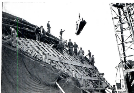
Near right: crane placing concrete in double forms from a hopper. Far right: strips of felt being mopped with asphalt to dome
