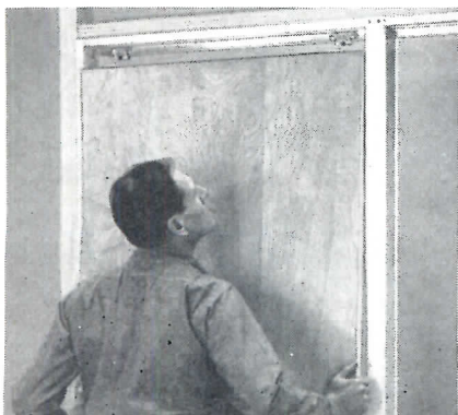
Time and Labor saved with this assembly line method of installation. Grant 7000 works beautifully, cuts costs!
