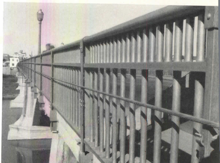
International Bridge, Laredo, Texas, has aluminum railings installed in 1935. In the event of floods, the entire railing can be quickly removed.
