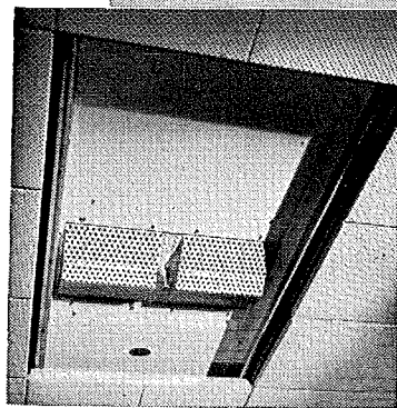
Concealed Multi-Vent Panel exposed by removal of six squares of metal acoustical ceiling.
