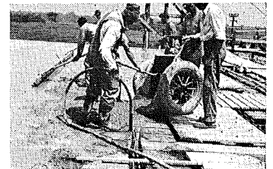
Concrete is being poured here over the steelforms and around the reinforcing steel. The final step is removal of steelforms and lumber after concrete sets.
