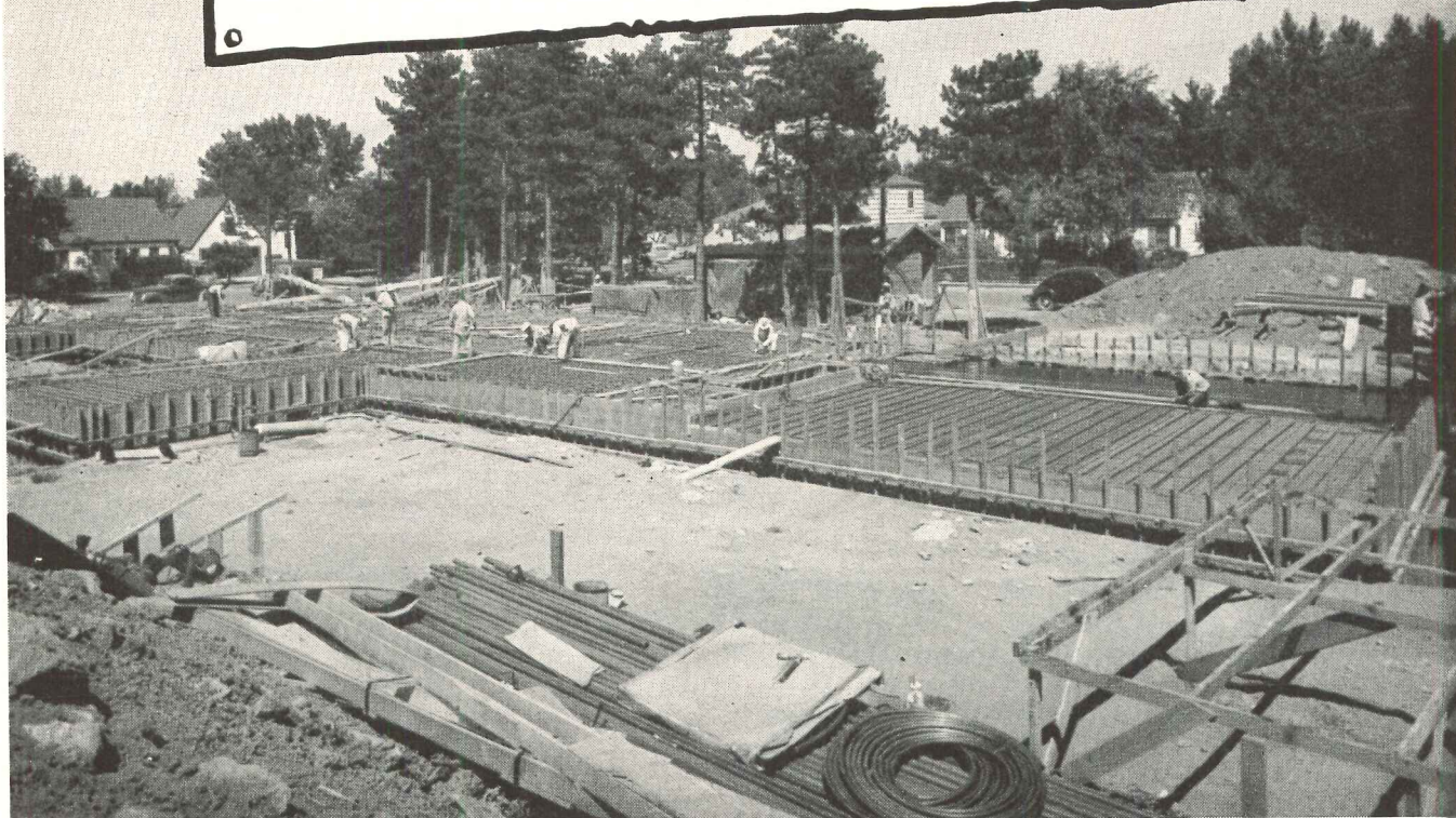
11,000 feet of Revere Copper Water Tube were used in the radiant panel heating system. The building has 9 zones, with each room controlled by individual thermostats. Revere Copper Water Tube was also used for hot and cold water lines, and Revere Sheet Copper for roofing.
