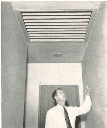
Pull on chain opens shutter and starts fan
