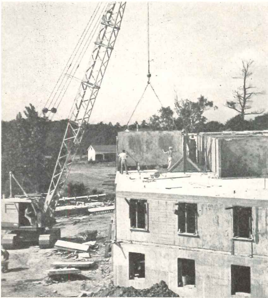
Photo, left: setting up precast wall slabs at the Univ. of Vermont. Simple wood bracing held slabs in place; floors were poured in place in forms built over slabs. Details below photo show typical dormitory construction. Bottom right: some of the first dorms built at the Univ. of Connecticut
