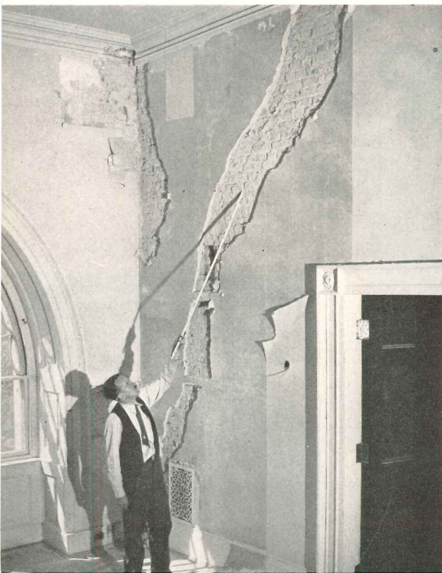
Plaster has been removed from one of the brick partitions to show settling cracks; these walls have no footings, were never intended to bear present loads
