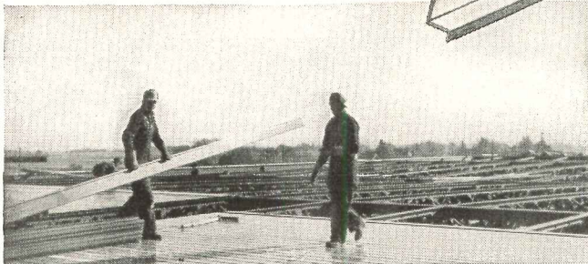
Truscon Ferrobord Steeldeck being installed in the new Automatic plant, Maytag Washing Machine Company, Newton, Iowa. Arthur H. Neumann & Bros., Inc., Des Moines, Architects, Engineers, Contractors.
