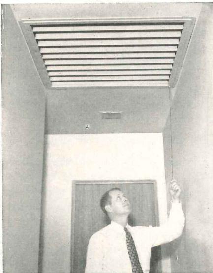
RESULT: cool comfort throughout entire house
