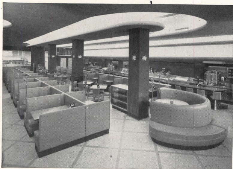
Clark's Restaurant, South Bend, Ind., features modern air conditioning system equipped with AAF Electro-Matic Electronic Precipitator.
