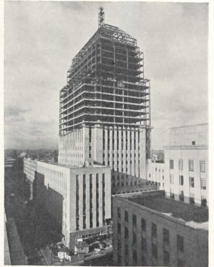
The 26-story office building for the John Hancock Mutual Life Insurance Company, in Boston. Cram & Ferguson, Architects
