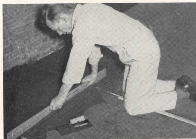
FIG. 3—Floor fill is mixed and applied to the floor like concrete topping. Wood screeds control thickness of the fill which is leveled with a straightedge. The surface of the fill is smoothed with a trowel and, where necessary, it can be troweled to a featheredge.
