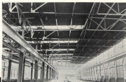
• Below: 1140 squares of Milcor Roof Deck were required to cover the huge Smith plant constructed as part of the national armament program.
