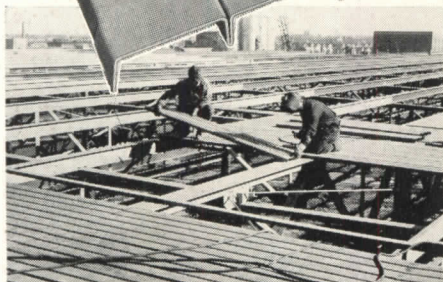
• Above: Milcor Steel Roof Deck being applied on new plant of A. O. Smith, Corp., Milwaukee, Wis.
