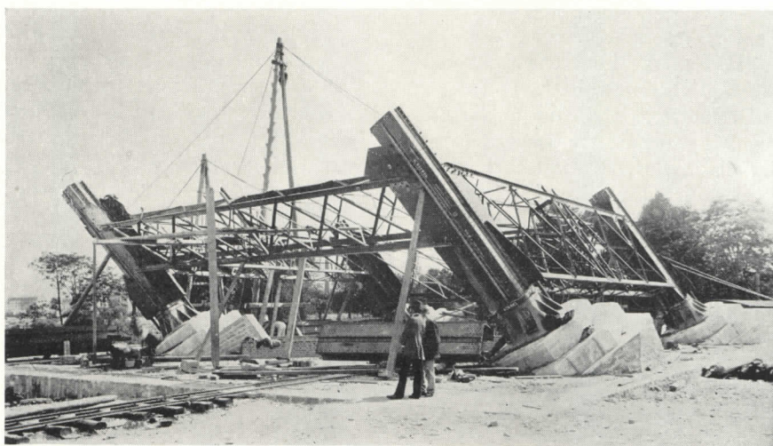
Fig. 6. Although worked in wrought iron, Eiffel's detailing of structural members would be quite adaptable to modern riveted steel construction. Photo taken July 18, 1887.
