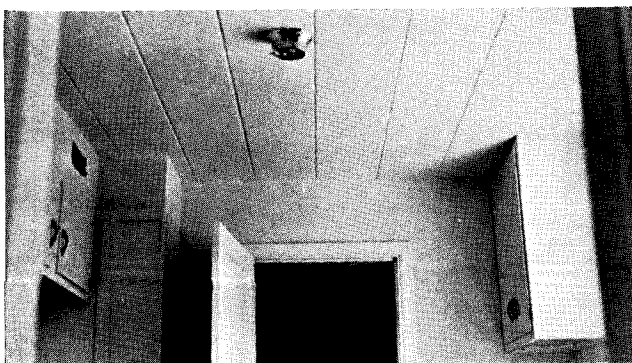
Fig. 29. The underside of the floor construction with hollow precast concrete units presents a smooth ceiling and may be finished by applying cement paint.
