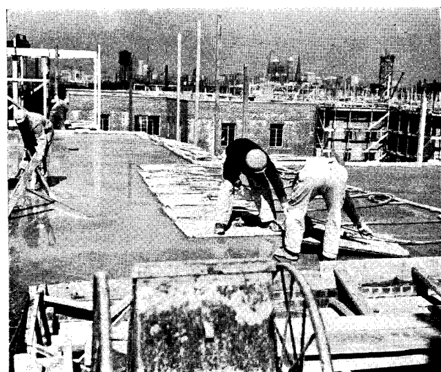
Fig. 5. Vacuum mats being used to remove excess water from concrete. After a 2½- to 4-minute application of the mats the slab is ready for finishing.
