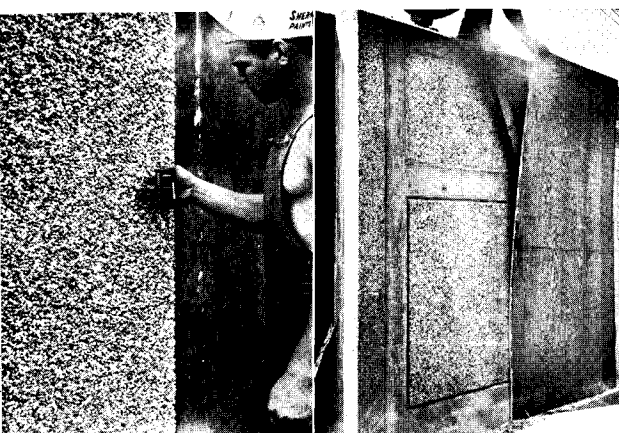
Fig. 17. Exposed aggregate surfaces for concrete walls by the bond-transfer method. Above, application of adhesive and aggregate to plywood form liner. Lower left, panels are attached to structural form with \frac{3}{4} -in. brads driven with a small brad gun. Lower right, structural forms are stripped; then liners are peeled off.
