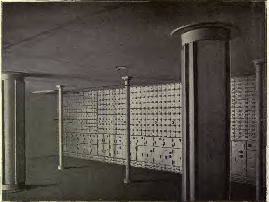
Fig. 3.—Interior of large vault shown in plan in Fig. 2. Of the safe deposit safes the larger lower ones are for the use of banks and large concerns, the upper and smaller for individuals. The two large columns are part of the construction of the building. The small columns will be removed when the rest of the stacks of safes are put in place.
